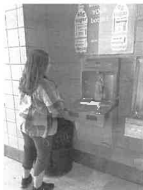
Hydration stations installed in Pipestone Area Schools.
